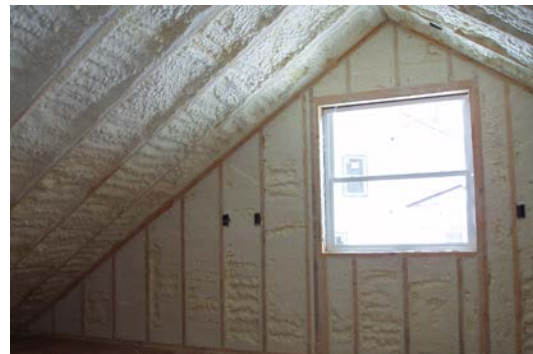
SPF insulation used in an attic space
